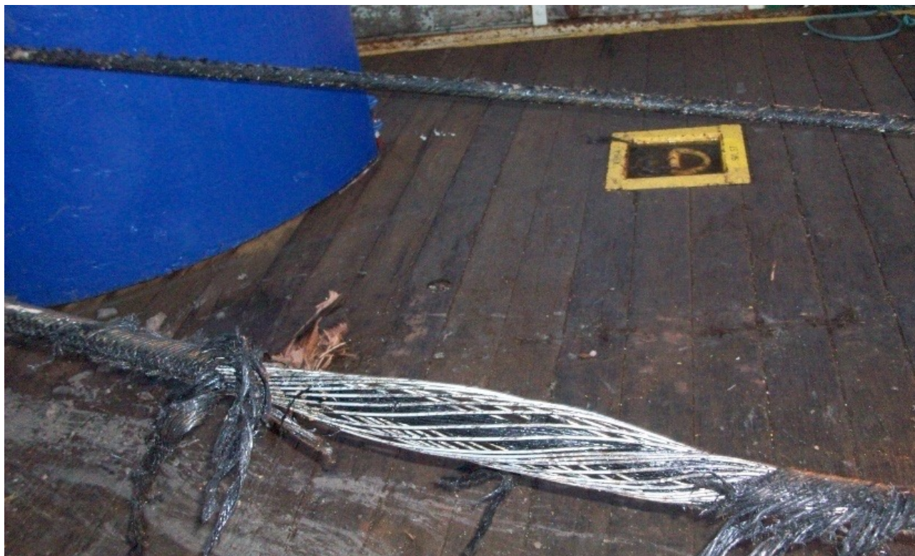
Figure 9. Damaged cable armor. Source: European Subsea Cables Association
